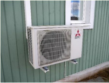
Figure 1 - Condenser unit of an ASHP
