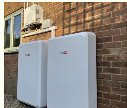
Figure 2: Household battery storage. Source: https://www.cahillrenewables.co.uk/services/battery-storage/
