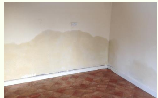
Signs of rising damp
