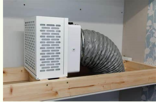
Positive input ventilation unit.
