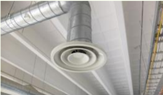
Mechanical extraction ventilation in an office
