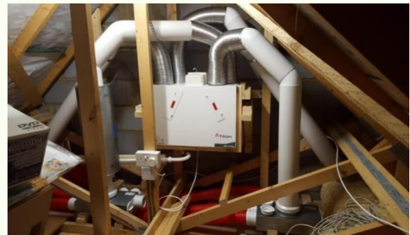
Heat recovery system installed in the loft.
