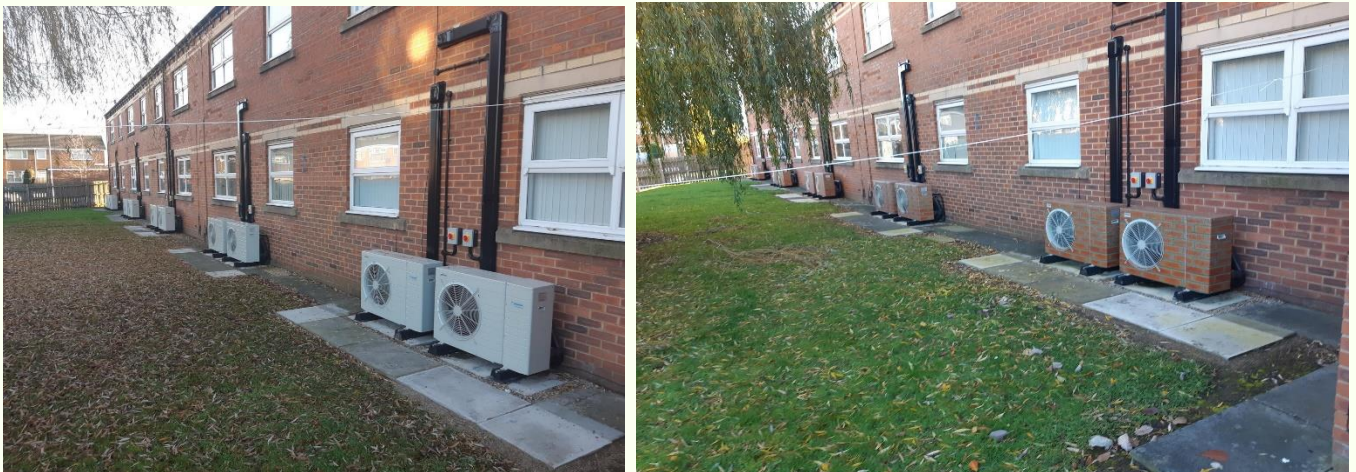
Figure 1 shows heat pumps before and after 'wrapping' so they complement the building and local area aesthetically. Source: Thirteen Group
