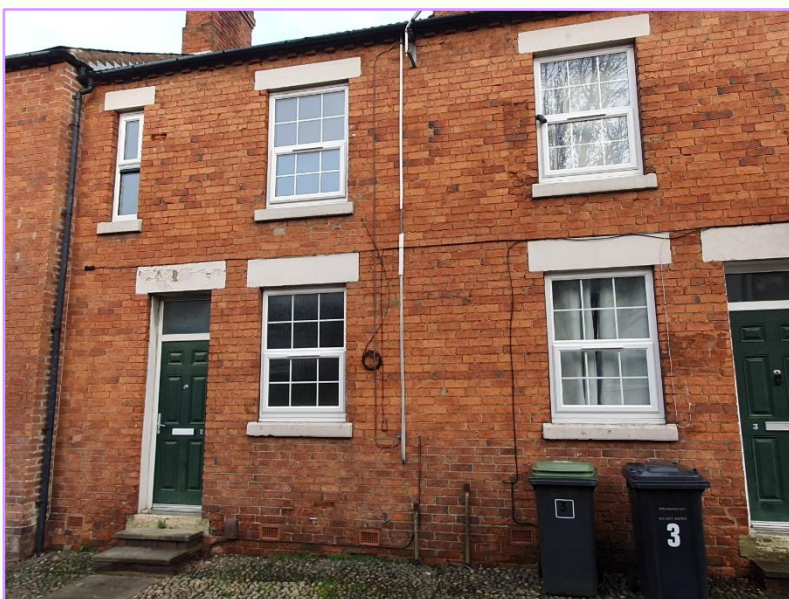
Figure 3: Before image of Princess New Street showing some degradation. Source: Broxtowe Council
