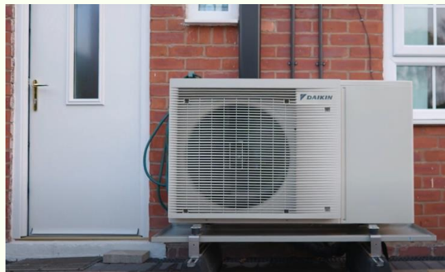
Figure 1: An Air Source Heat Pump, Source: Daikin
