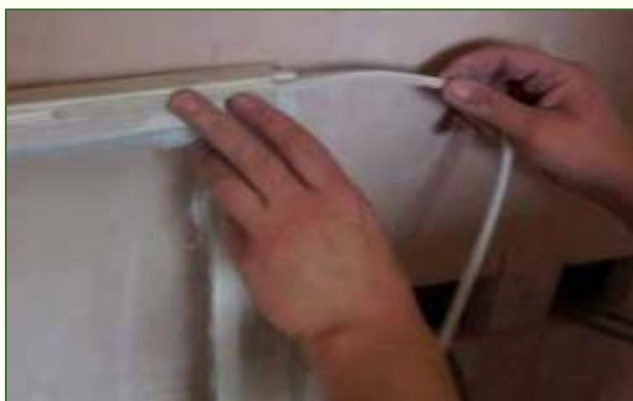
Figure 17 shows a nylon brush being inserted into a sash window as draught proofing. Source: Historic England.
